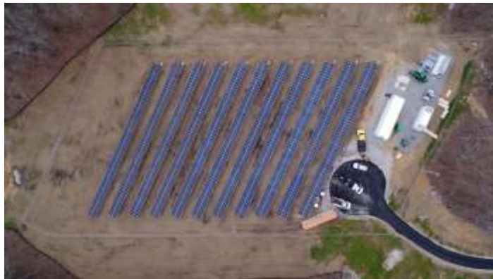
Front of the Meter DERs (Microgrid)
